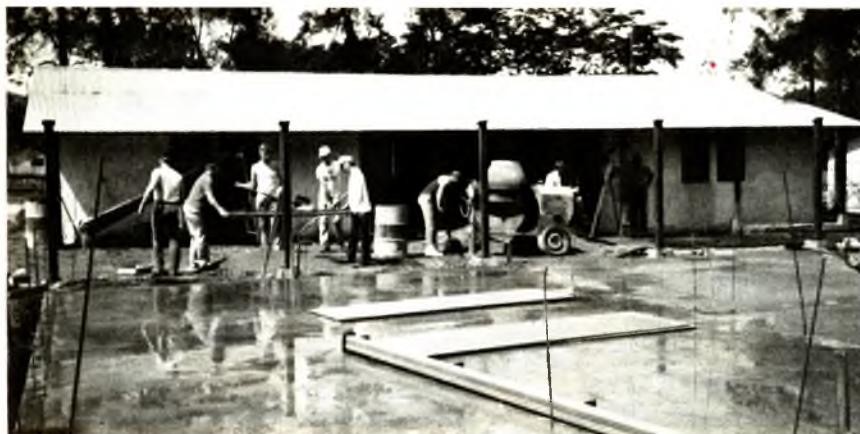
Members of the crew prepare to finish pouring the floor of one of the dorms. They are standing in front of one that had already been completed.
